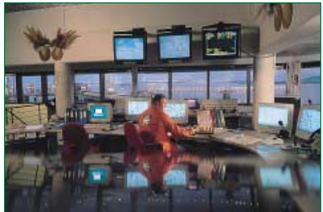
Scandinavian chic: the control room of the Sture oil terminal. ABB is modernizing the main control systems and integrating functions such as gas detection and emergency shutdown
